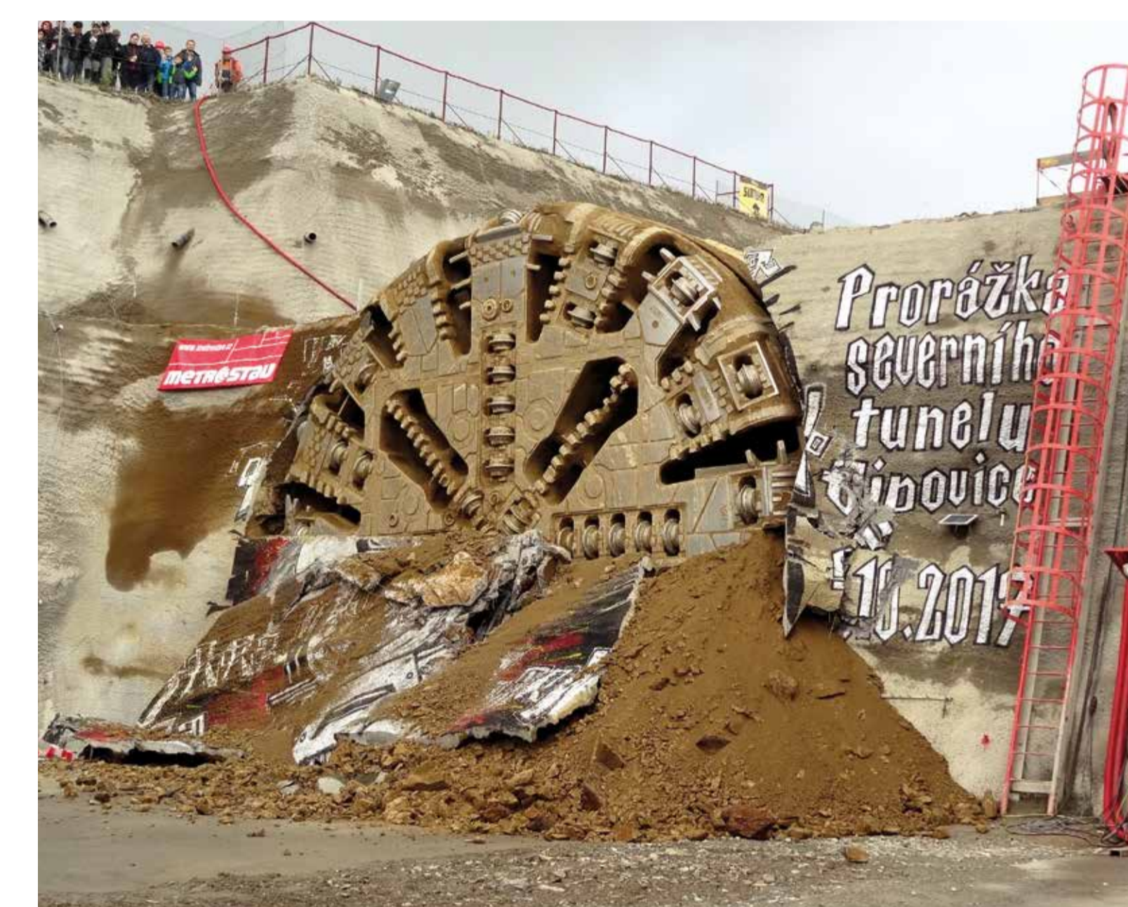
Prorážka severního tunelu Ejovice Breakthrough of the Ejovice northern tunnel, the Czech Republic
